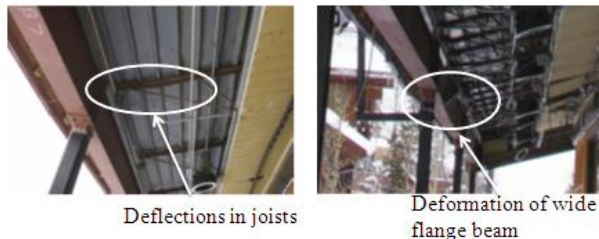
Figure 5: Deflected (a) bar joists and (b) wide flange beams due to large snow loads in February 2008 [11].
