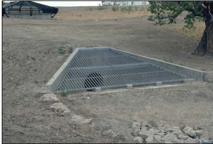
Photograph SO-6—Public safety is an important design consideration for detention facilities, including the potential need for safety/debris racks on outfall structures, as shown in this dry pond.
