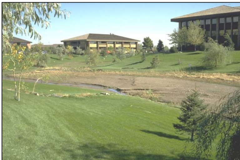
Photograph SO-8—Maintenance considerations must be carefully accounted for during design, with sediment accumulation a particular concern.
